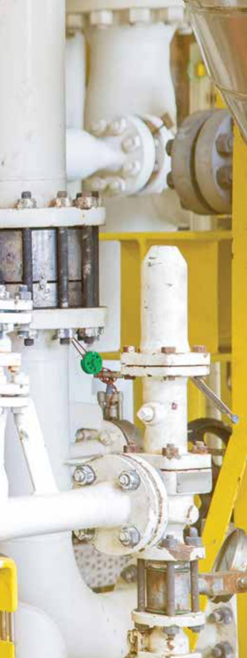
◀ Figure 1. An operator checks and logs the value of a differential pressure gauge.
